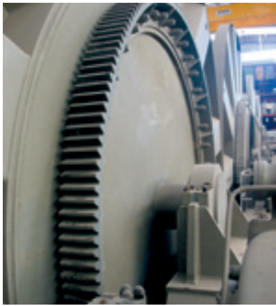
Intermittent lubrication with long intervals is the standard method for large open gears
